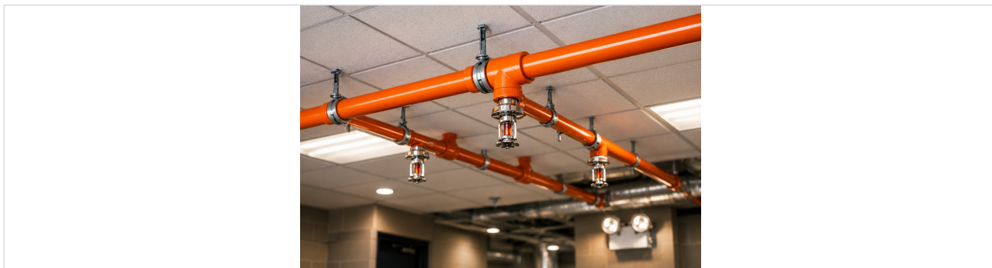
Orange CPVC fire sprinkler pipework — lightweight and fast to install, but vulnerable to chemical contamination from adjacent materials.
